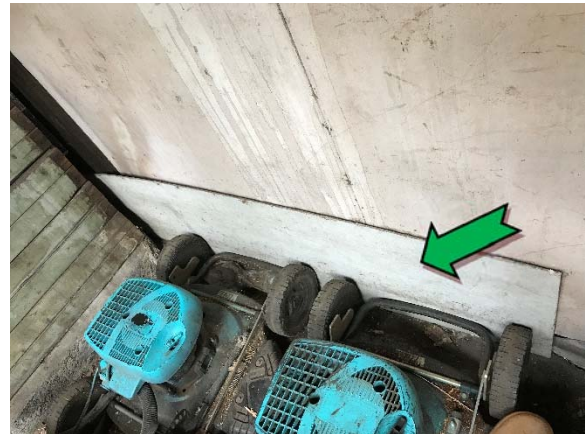
Photo 2. Interior, ground level, maintenance shed, south wall redundant panel – non asbestos-containing fibre cement sheeting.
