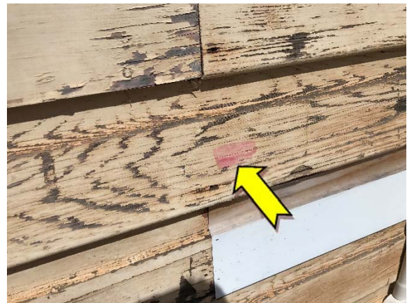
Photo 4. Exterior, throughout, walls – suspected lead-containing cream upper paint system.
