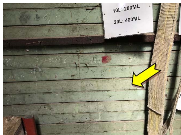
Photo 6. Interior, throughout, walls – suspected lead-containing green upper paint system.
