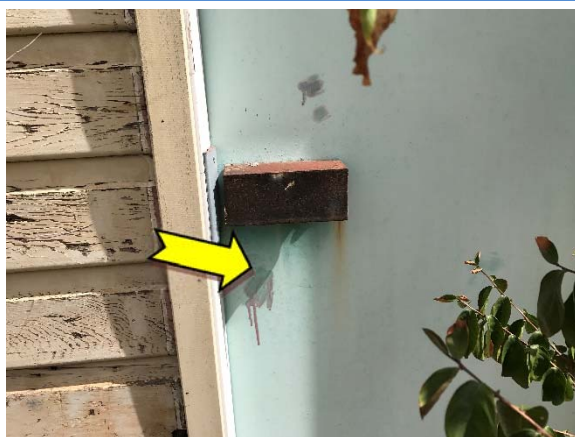
Photo 5. Exterior, throughout, doors – suspected lead-containing green upper paint system.
