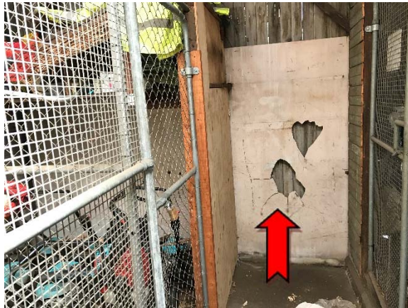
Photo 1. Interior, ground level, maintenance shed, south wall – asbestos-containing fibre cement sheeting.
